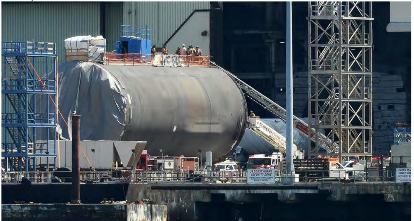
The scene of a fire Wednesday, July 27, 2022 on the future USS IDAHO on the docks at Electric Boat in Groton, Connecticut. (Dana Jensen/The Day)
